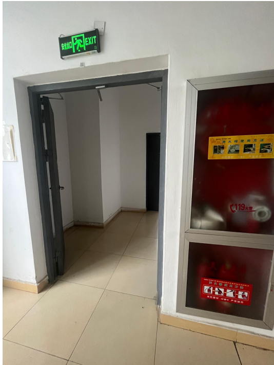
Dormitory fire exits and fire hydrants
