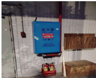
Fire extinguisher with inspection mark.
