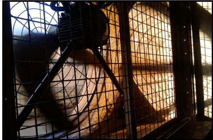
An oil-stained fan in the production facility
