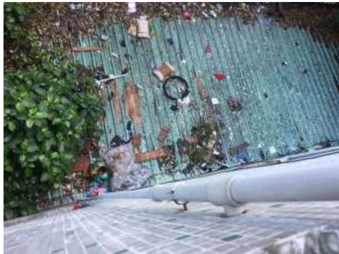
(Rubbish dumped outside factory)
