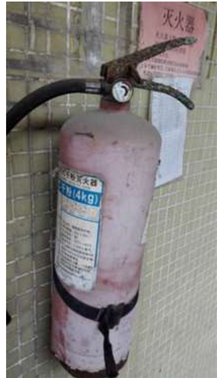
(A fire extinguisher in the factory)
