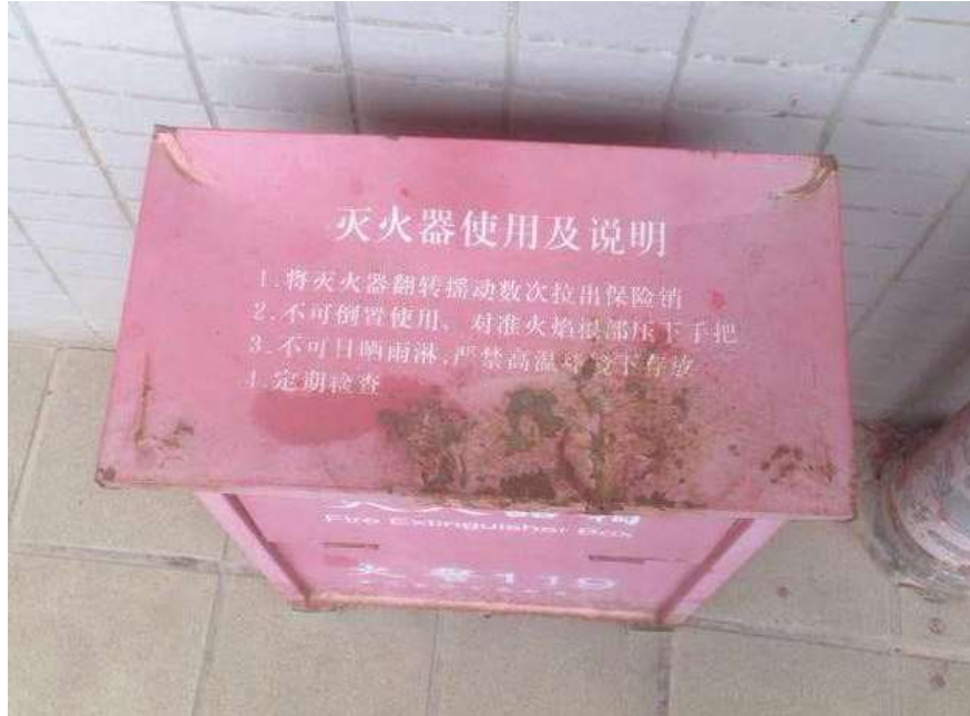
Fire extinguisher box in the dorm stairwell; article four states the fire extinguisher should be regularly inspected but no inspection log was present.
