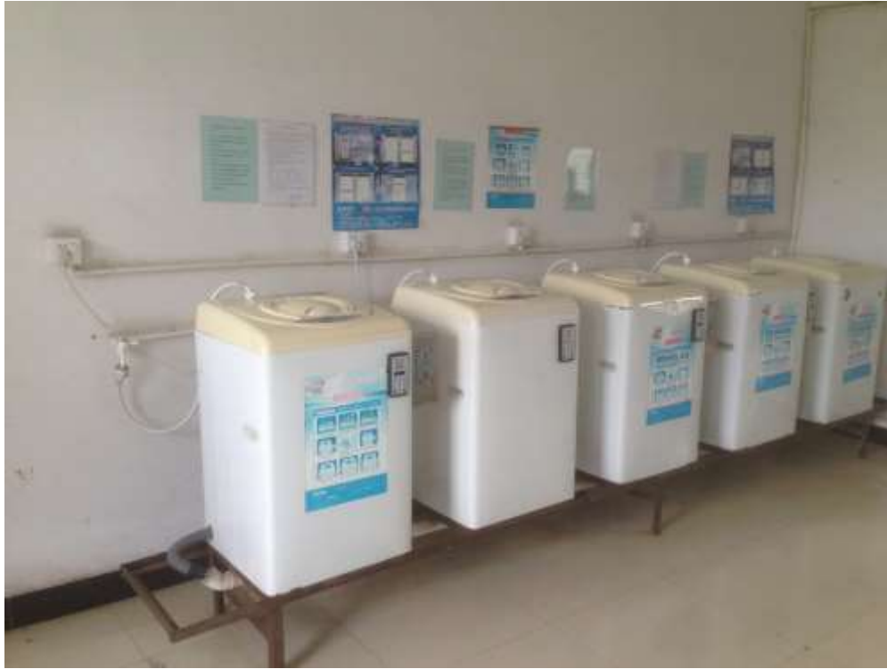
Washing machine room
