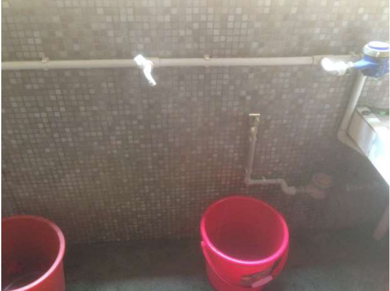
(Faucet on the balcony where workers fill up their containers with water)
