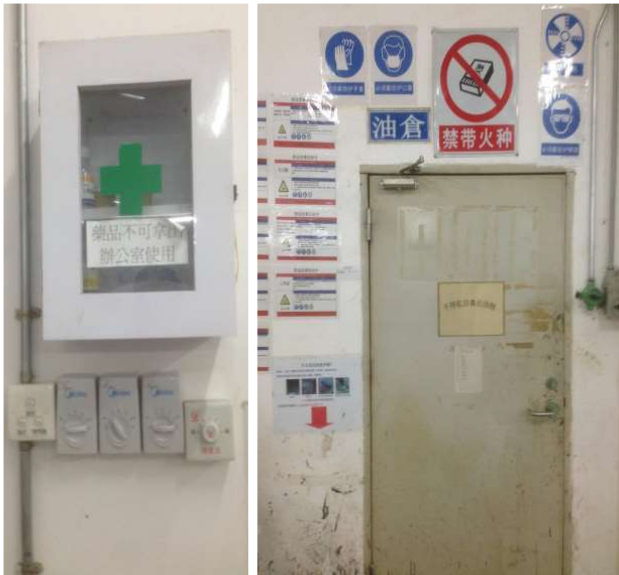
(Left: Emergency medicine box in the office with a sign taped to the front stating medicine should not be taken out of the office; Right: Oil storage facility with a list of hazardous chemical labels posted next to it as well as other safety notices.)
