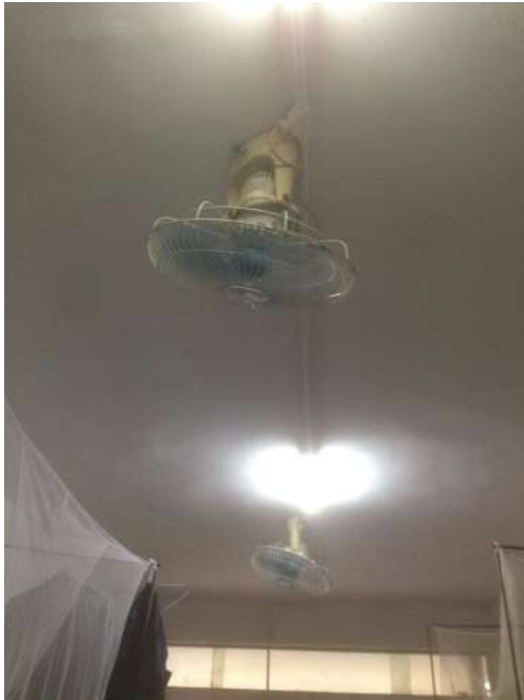
(Electric ceiling fans in the dormitory)
