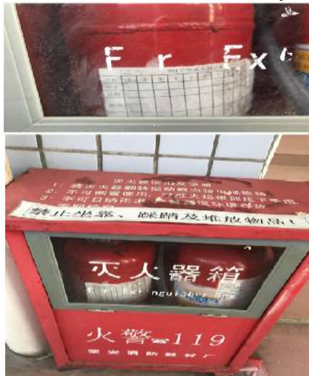
Fire safety equipment
