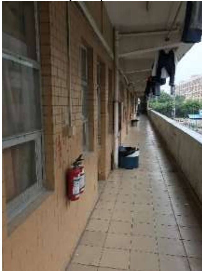
Dorm hallway is unobstructed
