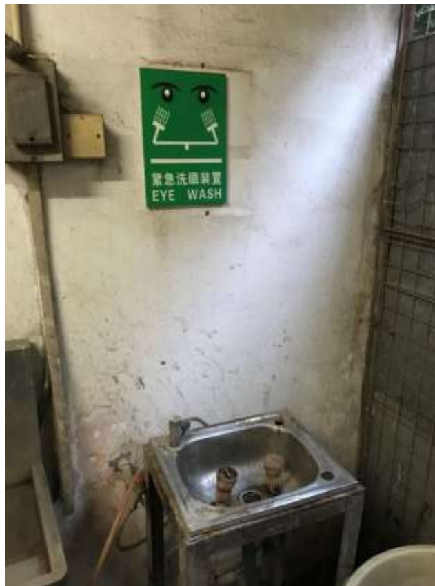
Emergency eyewash station
