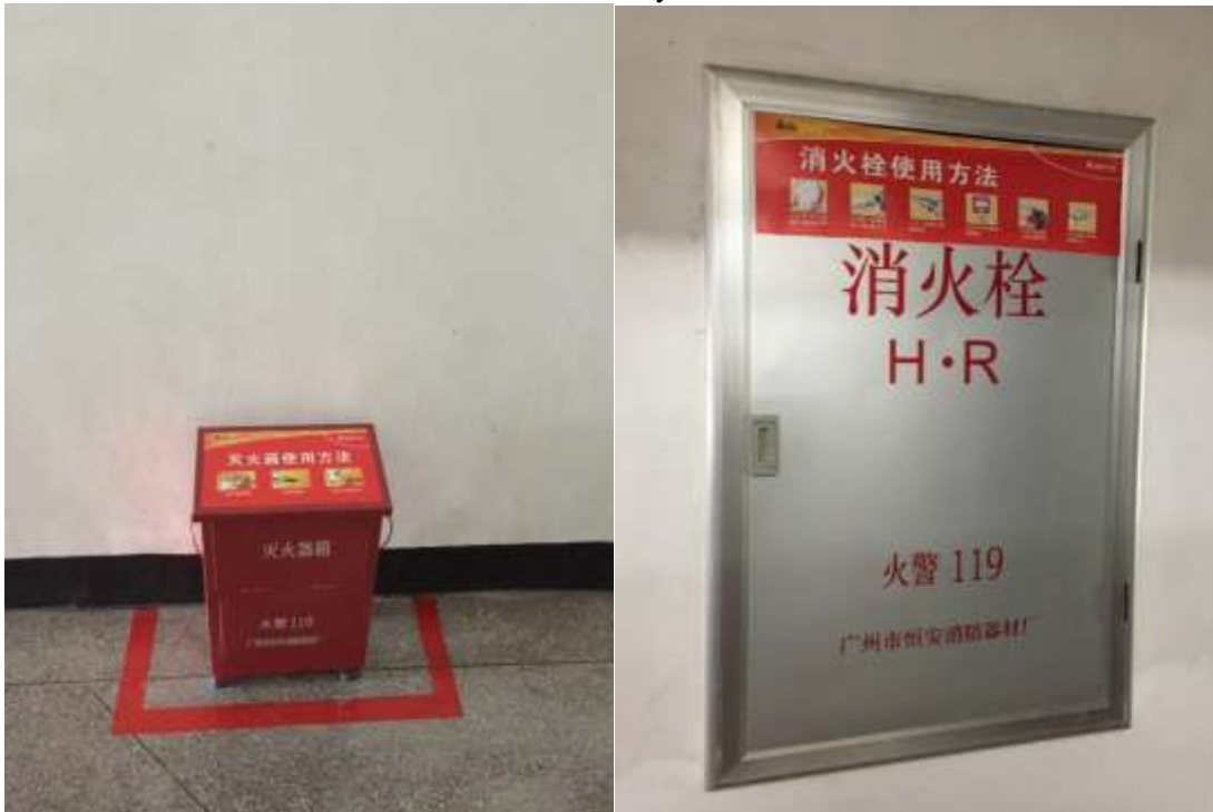
Fire extinguisher and fire hydrant located inside the factories
