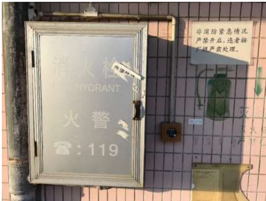
Fire extinguisher and fire hydrant
