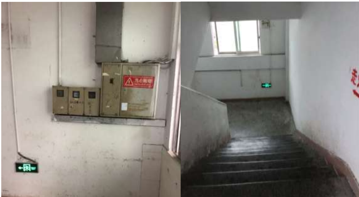
Emergency exit signs
