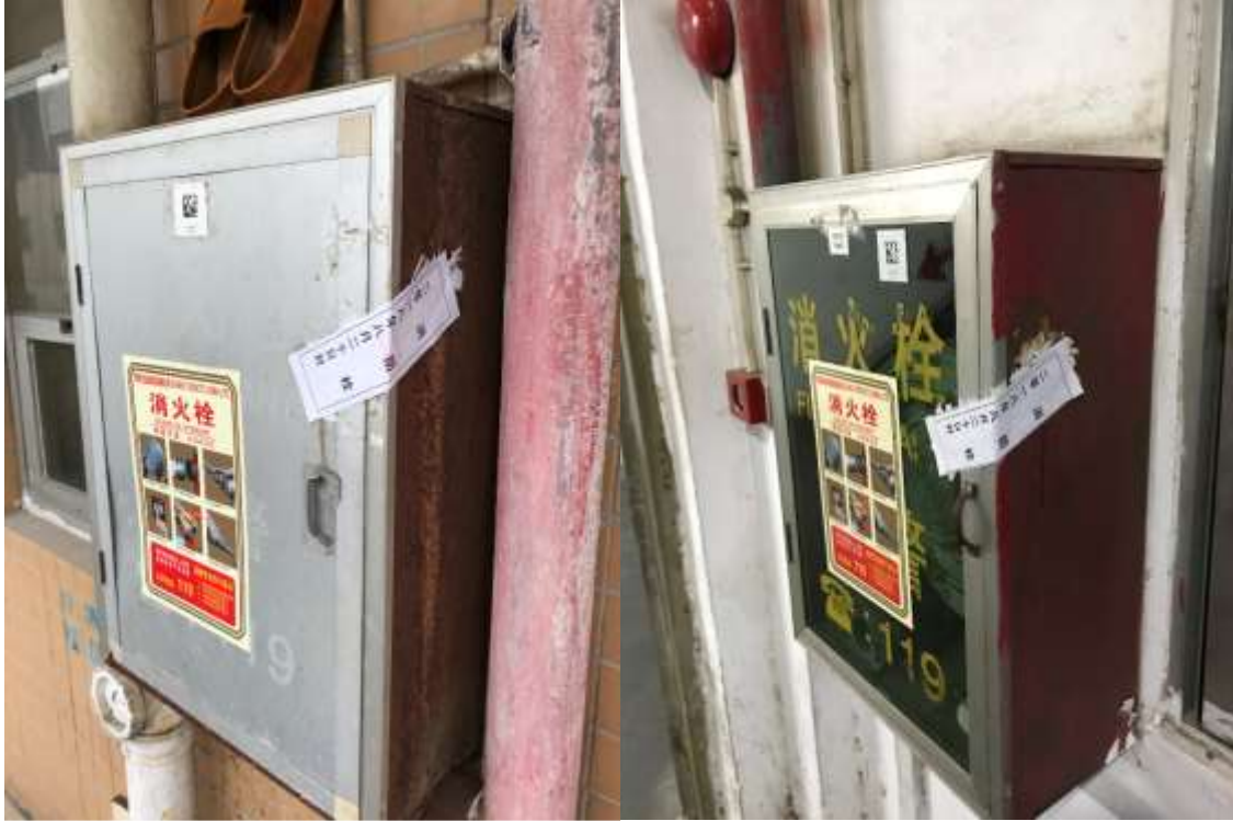
The fire hydrants in both the dorm and workshop had inspection log on it
