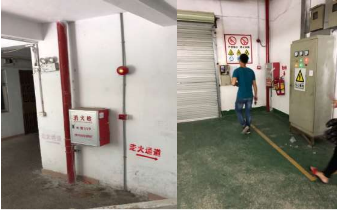
Left: fire hydrant and sign indicating where the emergency escape route is; Right: fire hydrant and fire extinguishers in the workshop as well as signage prohibiting smoking
