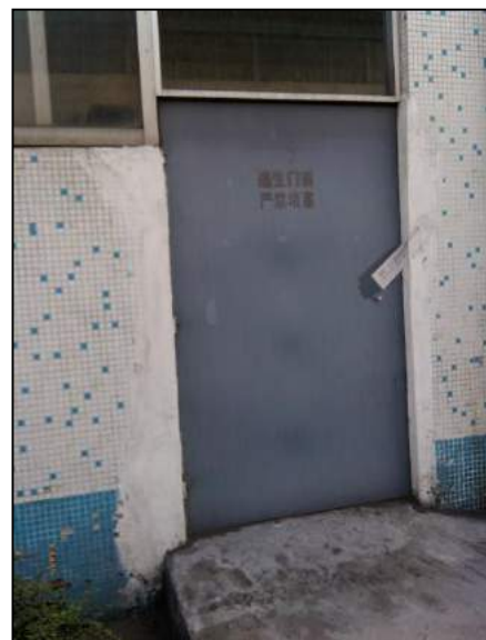
Locked emergency exit
