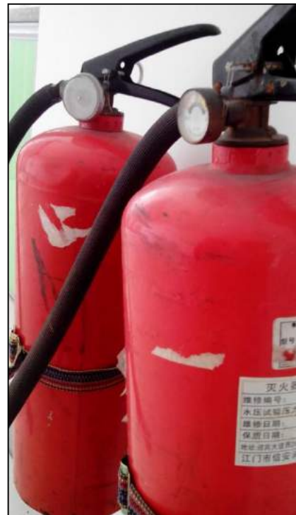
Old fire extinguishers without inspection records
