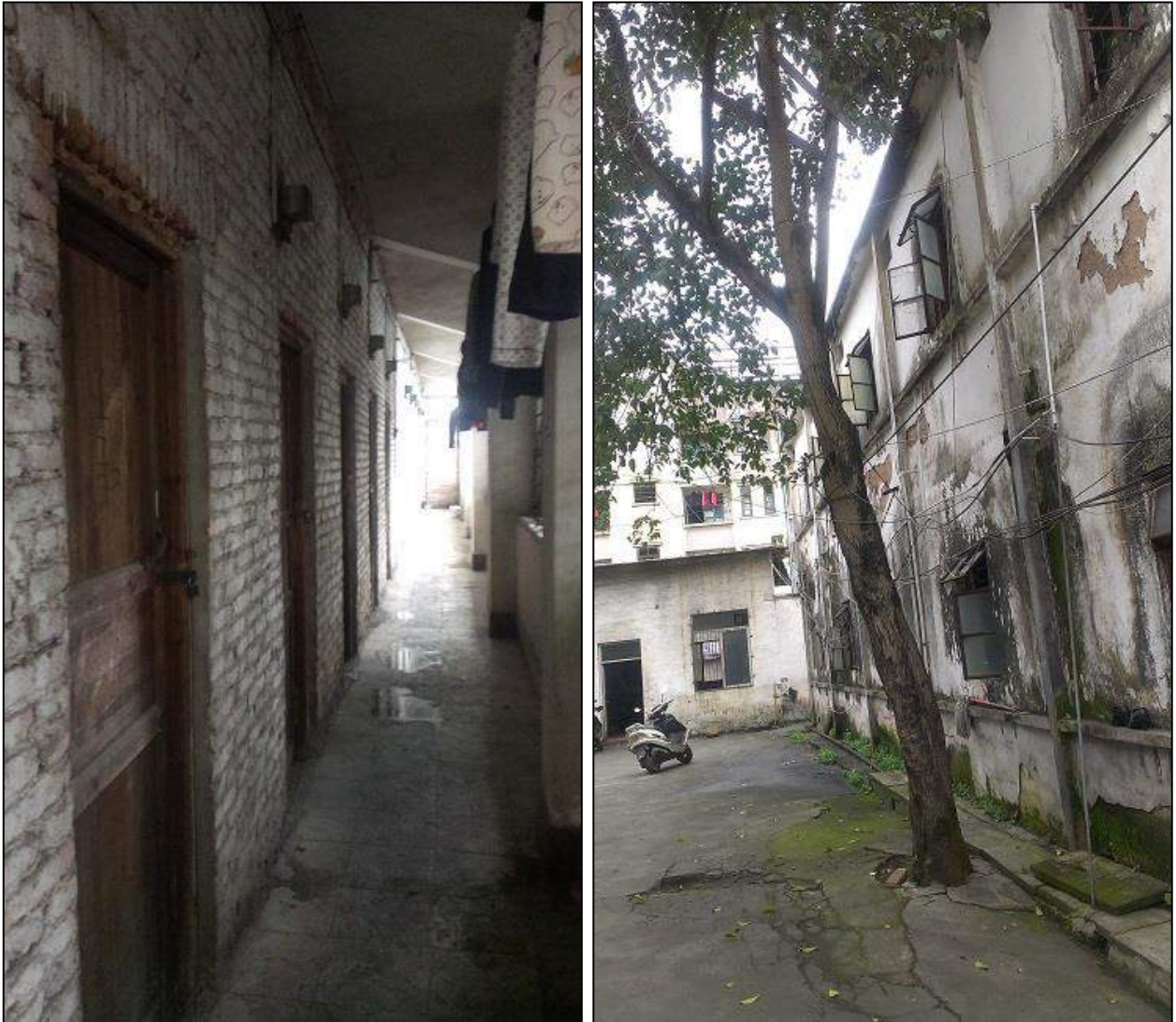
Left: Entrance to small rooms. Right: Many wires crossed and hanging outside.
