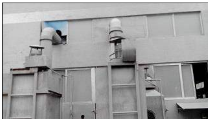
Dust from production is covers the outside of the factory building
