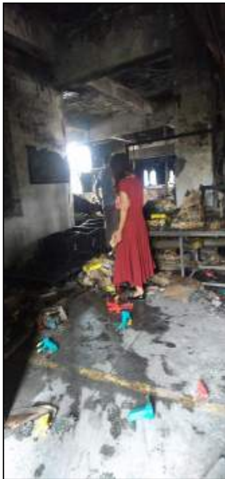
Management inspecting damaged workshop
