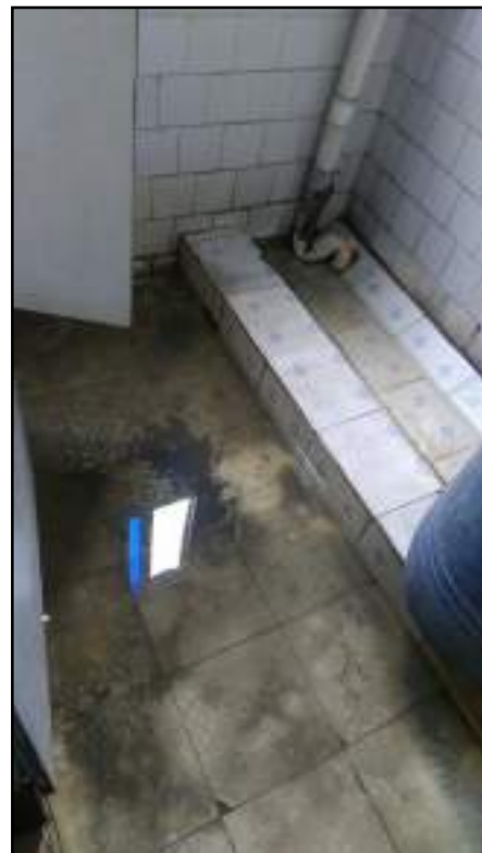
Water has accumulated on floor in one restroom
