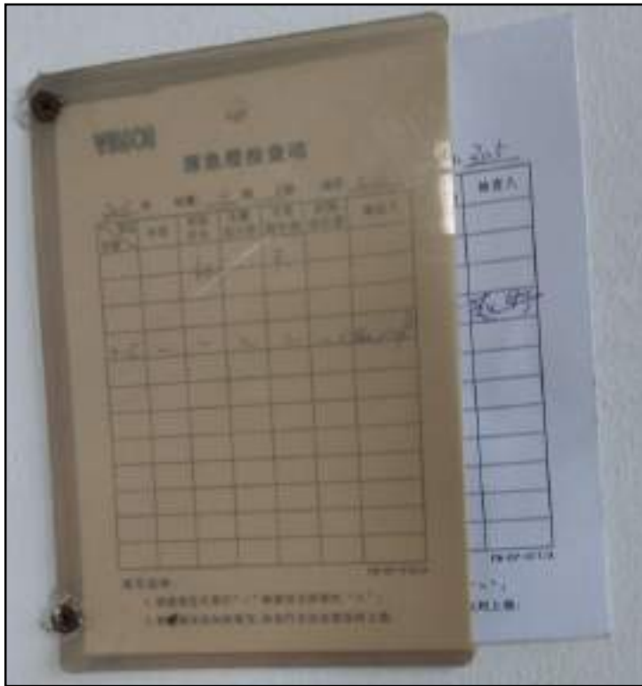
Fire safety equipment not regularly inspected
