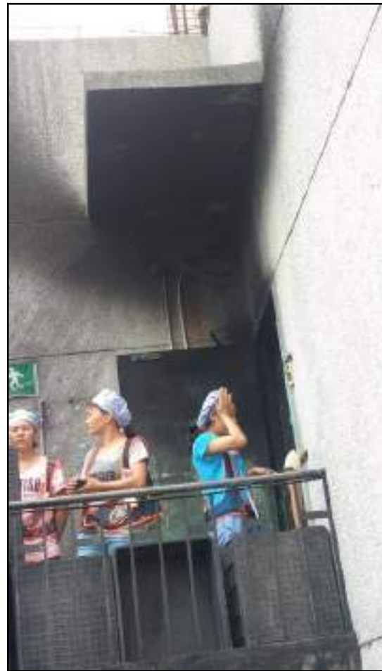
Burn marks outside workshop where fire occurred
