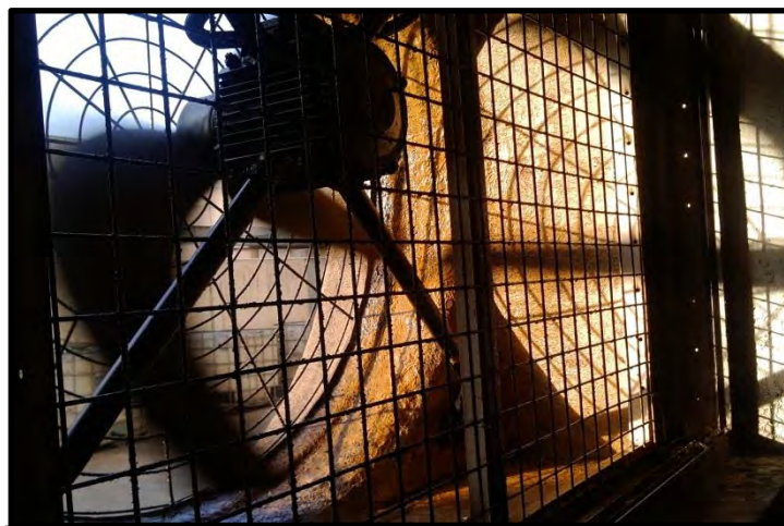
厂区内沾满油污的排风扇
