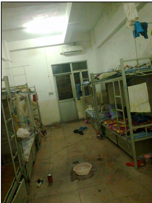
Basin used to catch water from leaky ceiling
