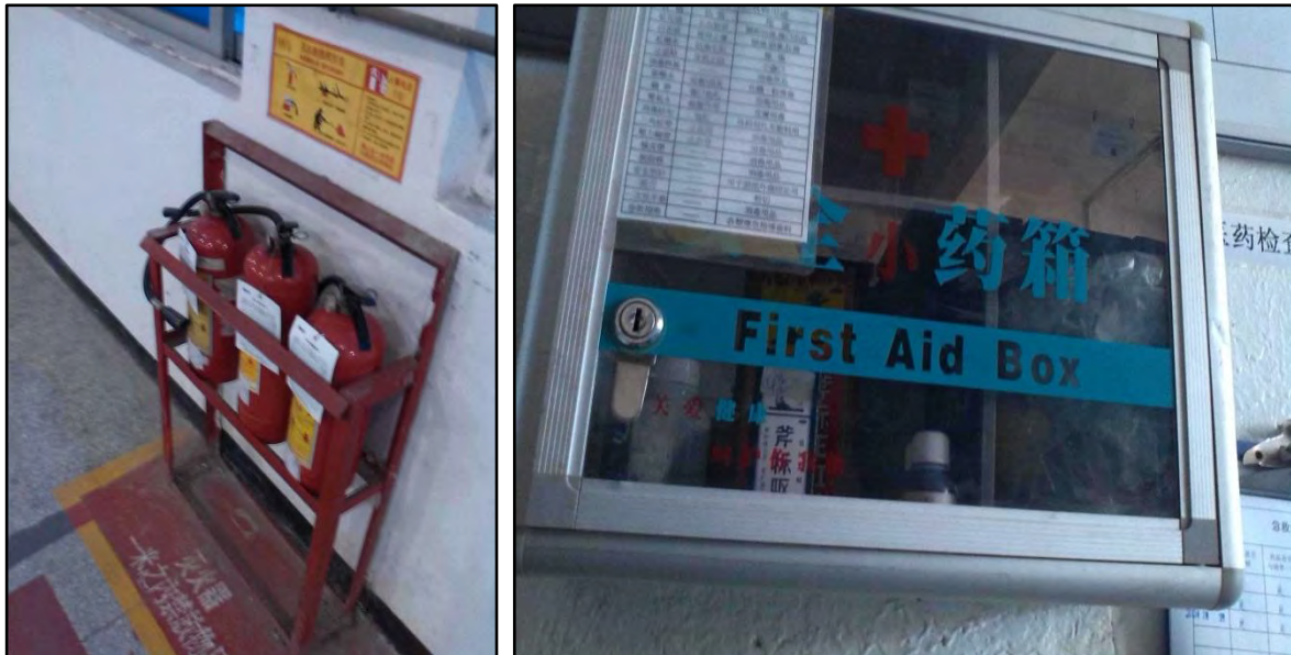
Fire extinguishers and first aid kit in production facility
