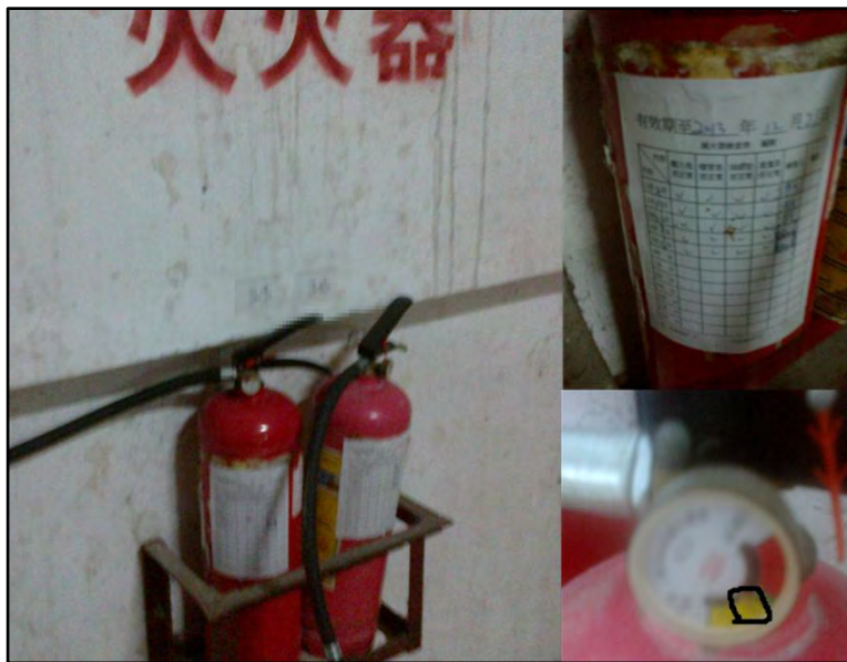
Over-pressurized fire extinguisher
