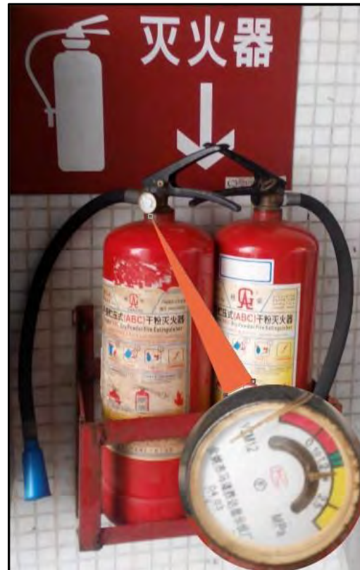
Overpressurized fire extinguisher
