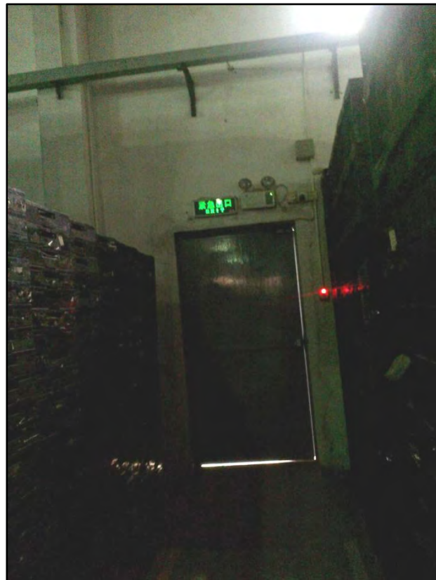
Emergency exit kept locked
