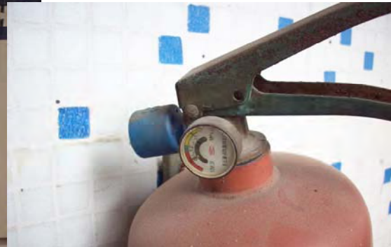
Image: Fire extinguisher found in Duoyuan, the meter pointed in red.
