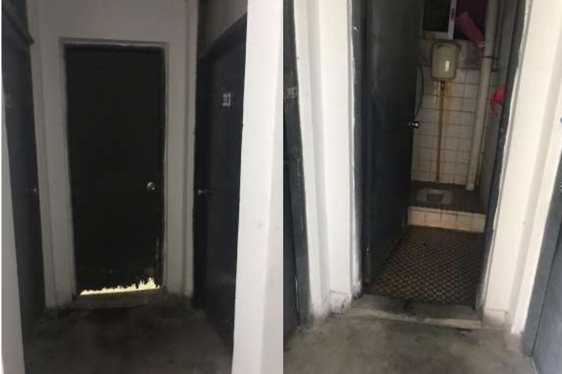
(Left: the bathroom doors are broken; Right: there is only one squat toilet in the bathroom)
