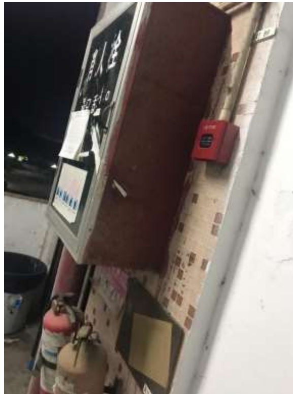
(A fire extinguisher in the corridor)
