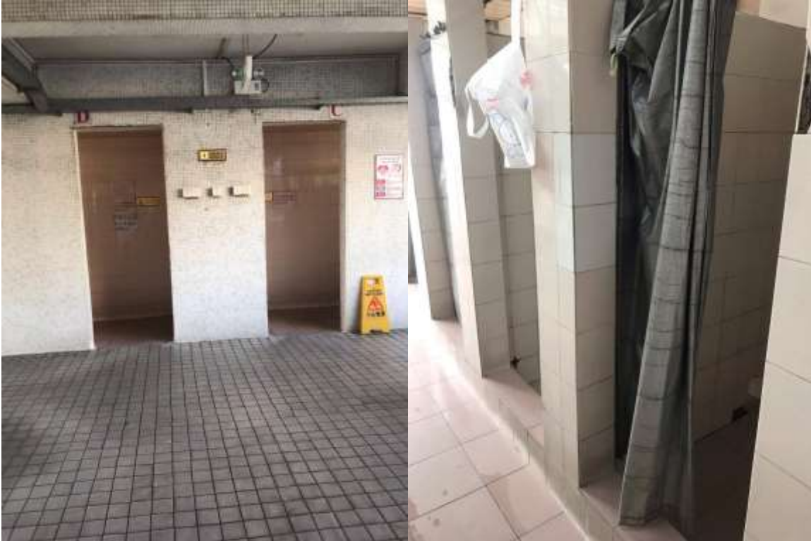
(Left: public bathrooms in the corridors; Right: there was no door and no privacy in public bathrooms)
