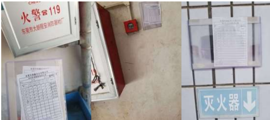
(Left: fire-call number and checkup list; Middle: fire alarm bell; Right: checkup list and a fire extinguisher mark)
